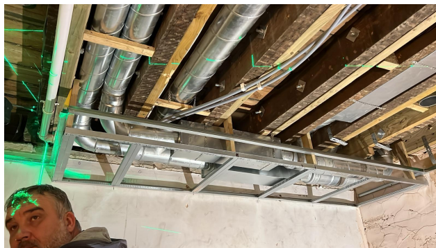
lowered ceiling portion for crossover & silencer in dining room (bath & shower rooms in phase 2). Most ducts are within joist space
