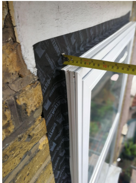
new windows, set forward to allow for EWI. External airtight tape for weather-seal
