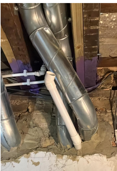
ducts passing from dining room into kitchen through wall (with condensate drain)
