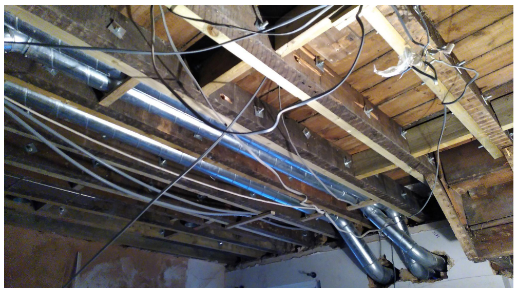
supply ducts for kitchen and bed 3, and extract from bathroom and kitchen passing through wall
