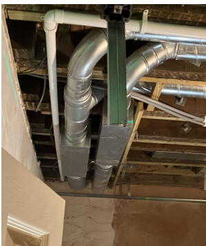
supply & extract ducts for kitchen & bathroom below joists
