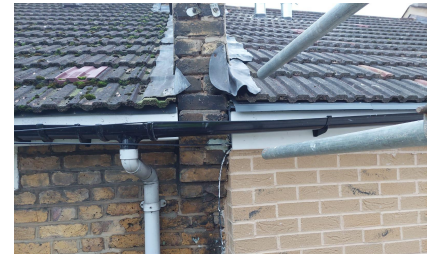
front elevation (NE) insulation short of party wall mid-line
